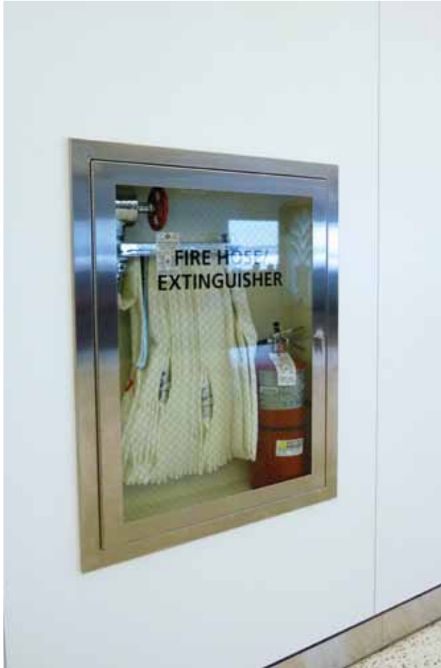
Recessed Fire Hose and Extinguisher Cabinet
