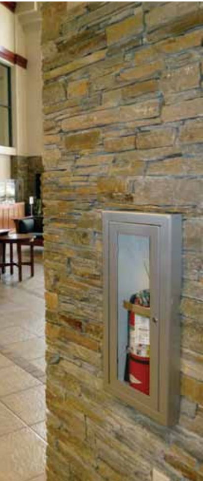
Semi-Recessed Fire Extinguisher Cabinet
