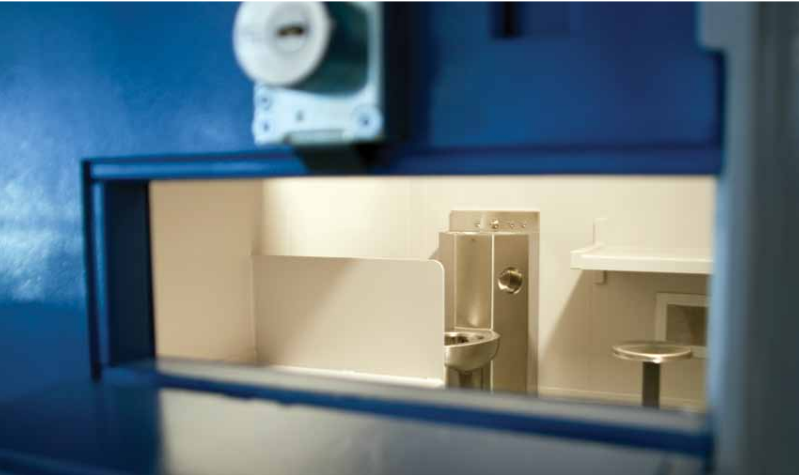
Stainless Steel Lav-Toilet "Comby" installed in a prison cell
