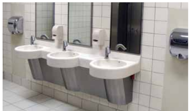
Acorn Engineering's Kurve® Basin reduces water consumption in a school setting
